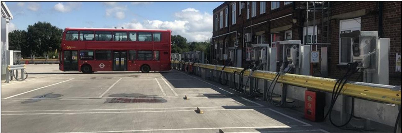
Figure A-3: Northumberland Park electric bus depot
