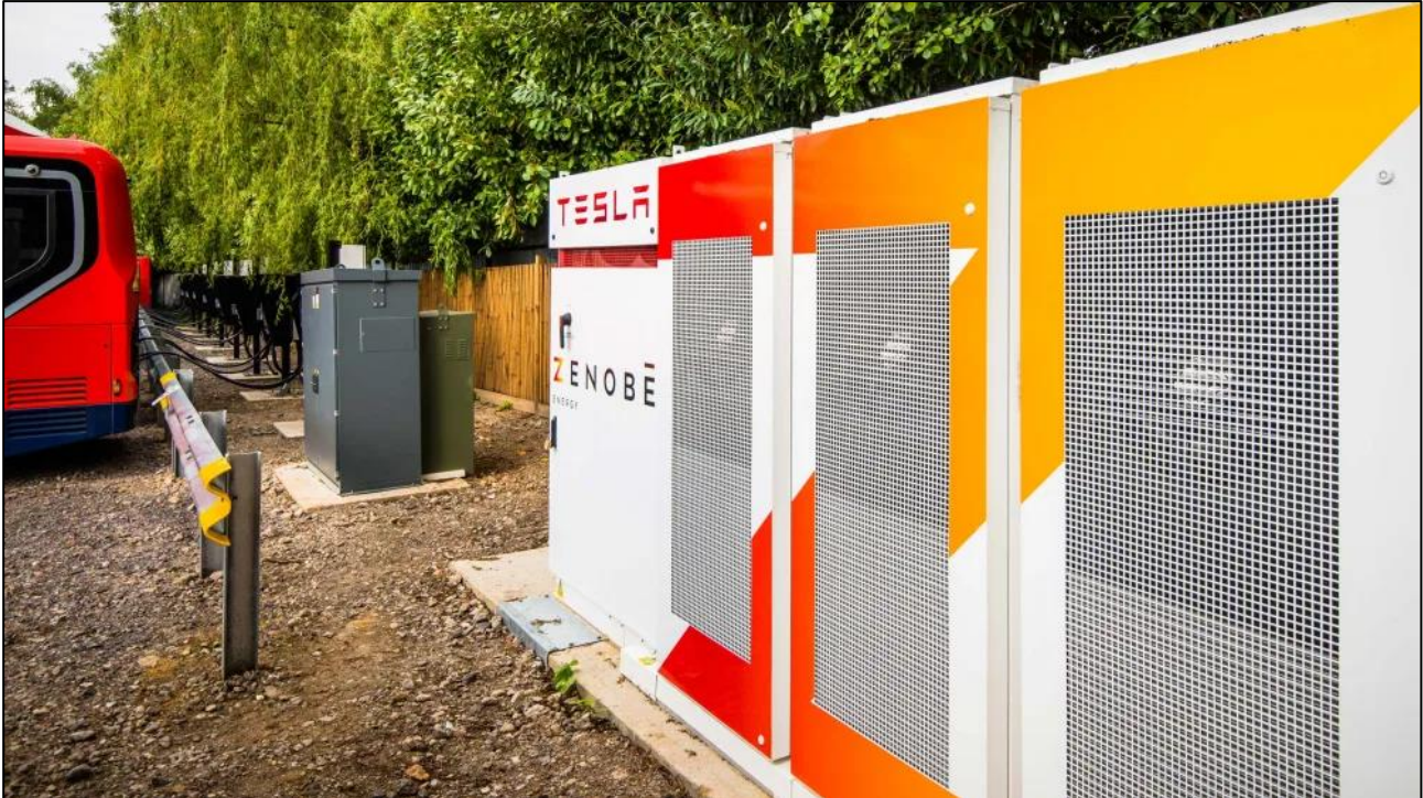
Figure A-2: Tesla Powerpack (78 units) installed at Stagecoach's Guildford Dept
